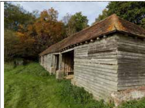
Figure 40: View of the southern elevation of the building on site showing the open sections of the building.
