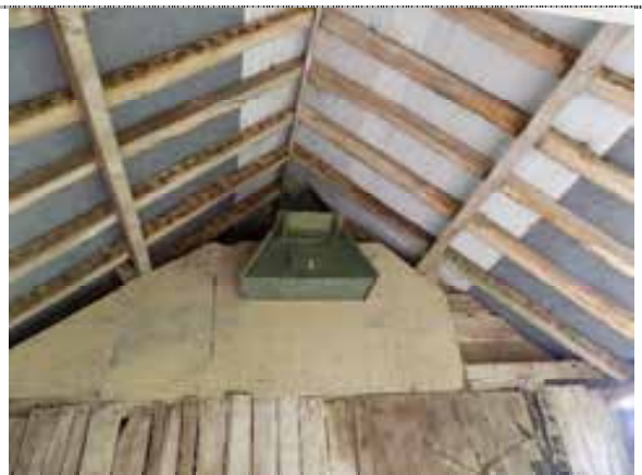
Figure 43: View of the roof structure showing the use of breathable membrane and an owl box located within the barn.
