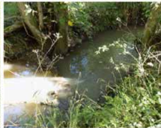
Figure 39: View of the same watercourse showing the high levels of sediment loading.
