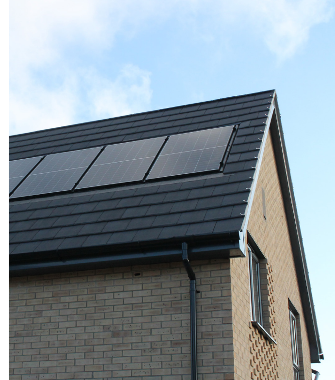
Solar Panels at our Ockford Ridge Scheme
