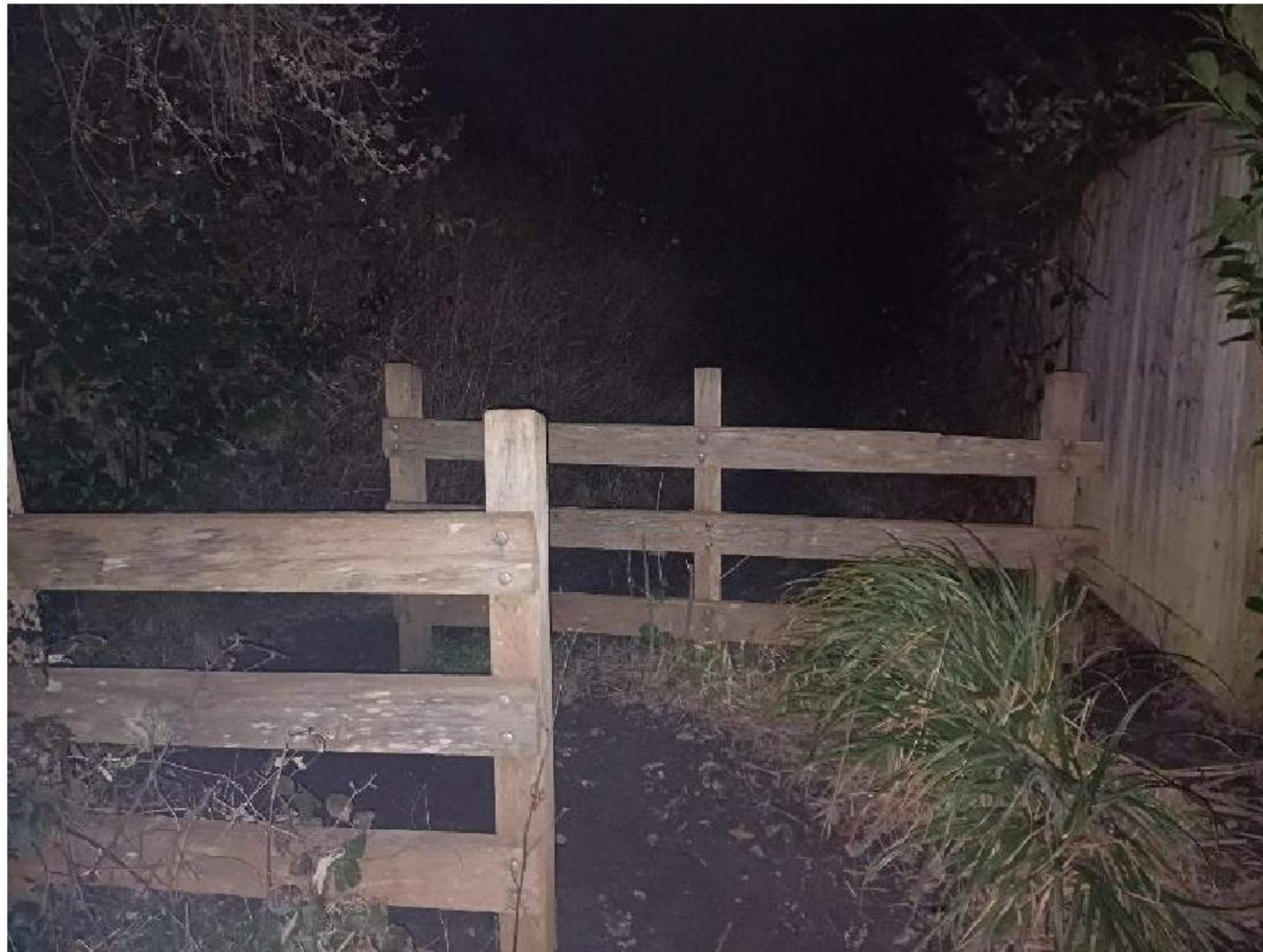
Figure 5: Uneven sections of 29CU footpath
